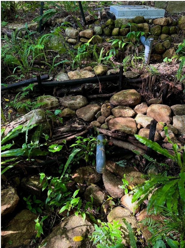
A wastewater garden: infrastructure integrated with stone, ground and fast-absorbing plants. Photo: Bobby Anderson.
